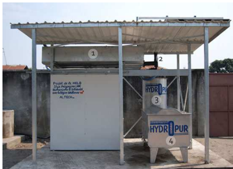
FIGURE 3. STATION HYDROPUR DE ALTECH SAFS
